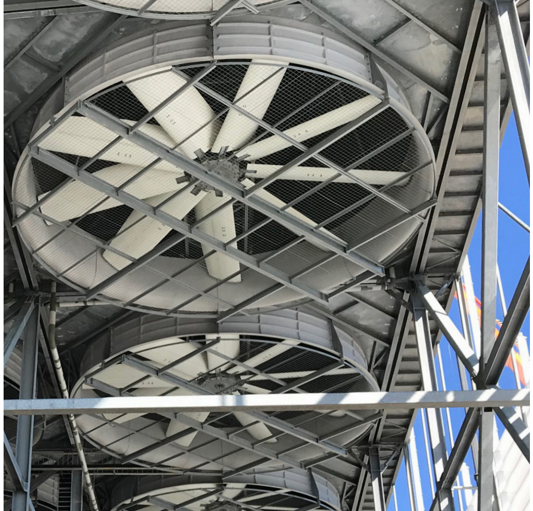
36' FRP Fan for ACC - Power Plant
