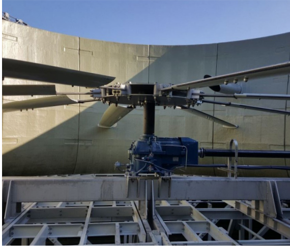
28' FRP Fan for CT with aggressive environment - Geothermal Plant
