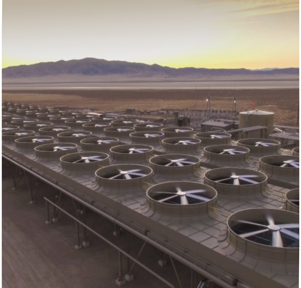
24' Aluminum Fan for ACC - ORC plant
