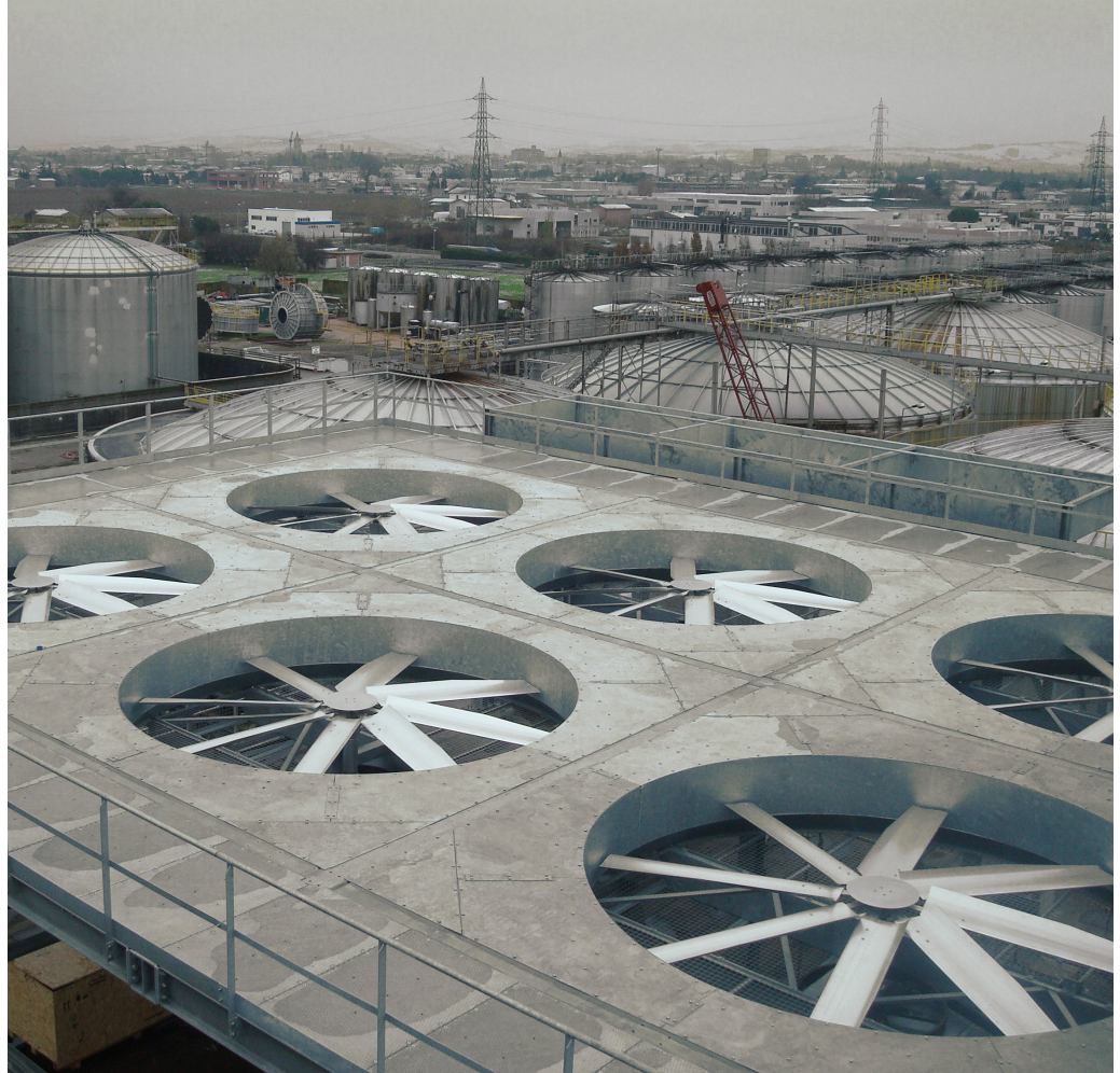
16' Aluminum Fan for ACC - Distillery Plant
