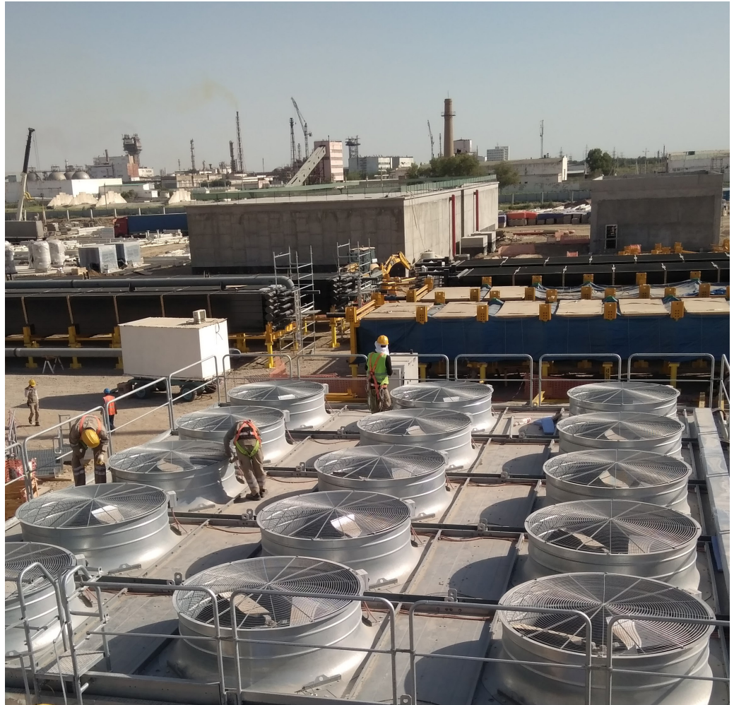
6' Aluminum Fan for AFC - Petrochemical Plant
